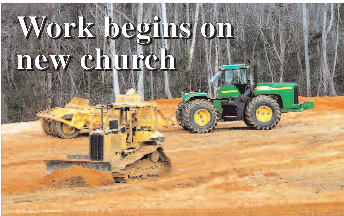
Choctaw Sun photo by Tommy Campbell GILBERTTOWN — Pastor Doug Chapman and the members of Gilberttown Assembly of God Church are celebrating the beginning of the construction of their new sanctuary. Site work got underway late last week, and by Wednesday of this week, the large hill behind the current church — where the new sanctuary will soon start to take shape — had been leveled. The church is located on Ala. 17 on the south side of Gilberttown. Watch the Sun in the weeks ahead for more information on the building project.
