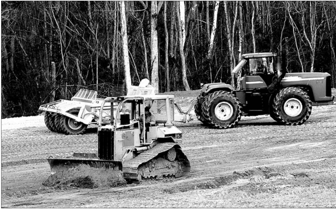
The land where the new Gilbertown Assembly of God Church is being cleared to get ready for construction, which is set to begin in 3 to 4 months.
