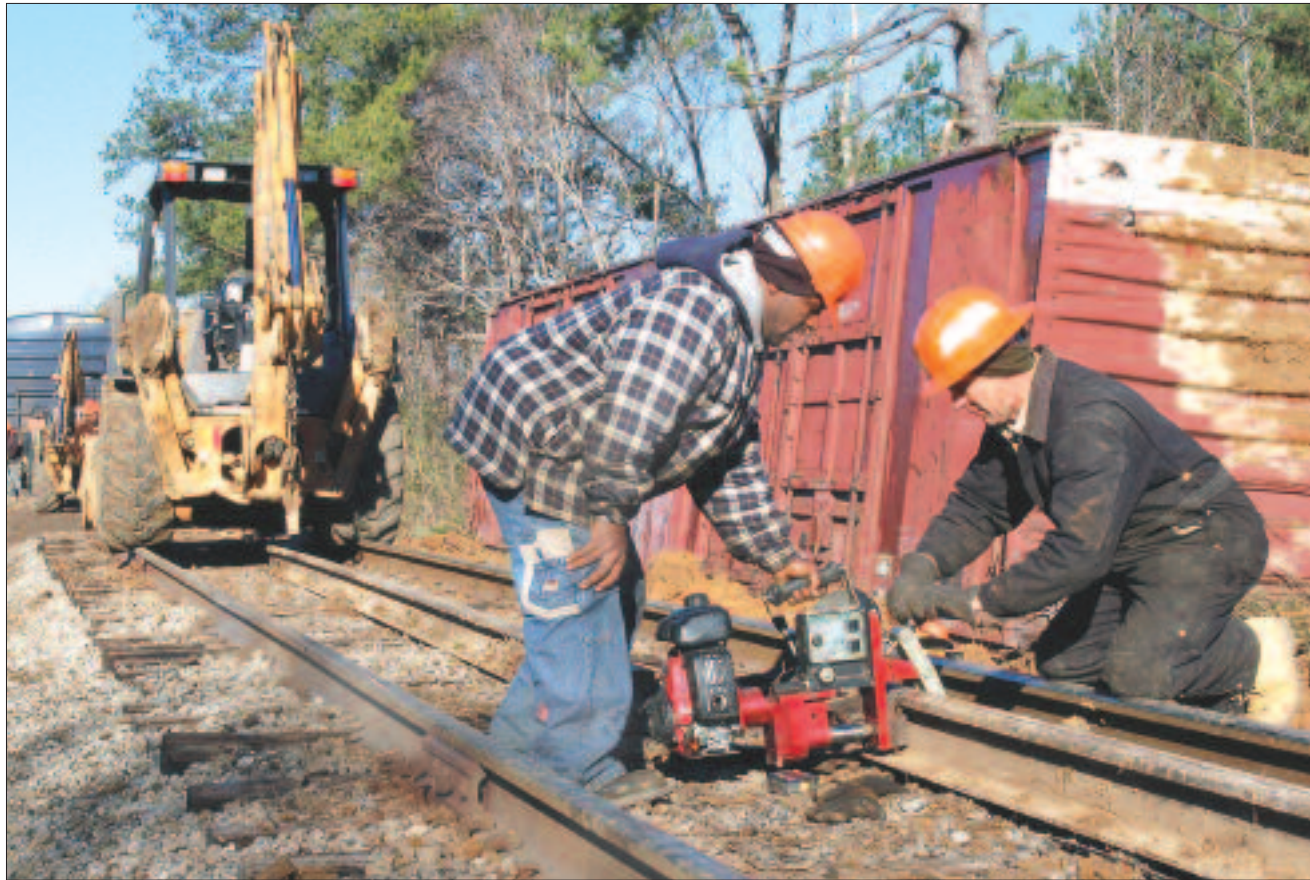
Photo by Tommy Campbell/The Choctaw Sun Andrew Lewis, of Dixons Mills, Ala., and Mike Nelson, of Wetumpka, Ala., employees of D.R. Davies Railroad Construction Company, are shown here early Monday morning in 20-degree weather repairing the railroad bed which was damaged when a parked M&B freight train suddenly started rolling and smashed into another set of parked cars a mile and a half down the track.
